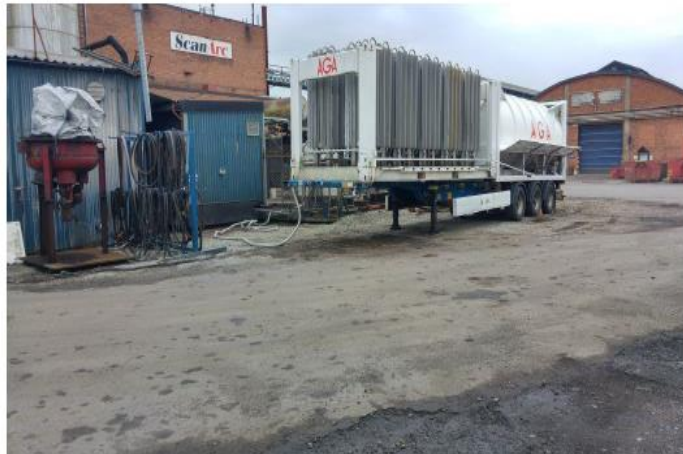
Figure 1 CO 2 tank with condenser outside Scanarc pilot plant.
